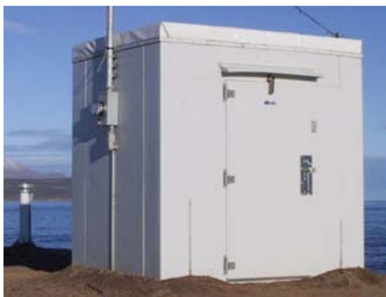
Figure 6. Tide Gauge Shelter with GPS Antenna, Qikiqtarjuaq.
